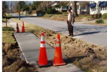
A section of sidewalk at 4th Avenue West is repaired as a part of Walk Wise, Drive Smart . The sidewalk is part of the "Walk Across NC" walking route near the Sammy Williams Center for Active Living.
