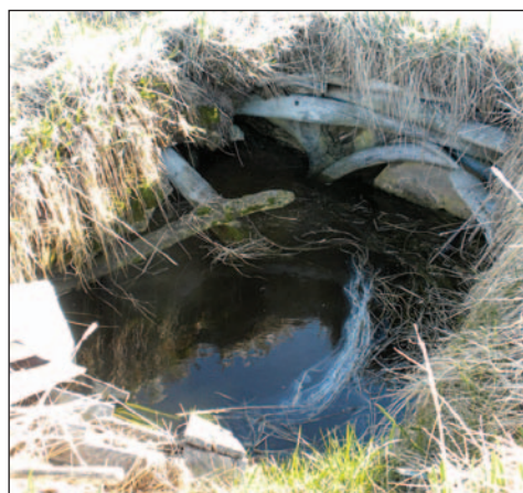
Flooded ice cellar. Mike Brubaker, 2010
